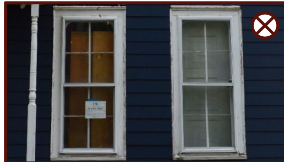
Figure 63: Example of an inappropriate modern window replacement that does not fit within the original wood casing on a historic residential building.
