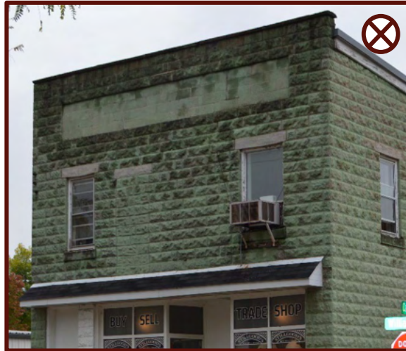
Figure 118: Example of inappropriately located AC unit on the front façade of a commercial building.
