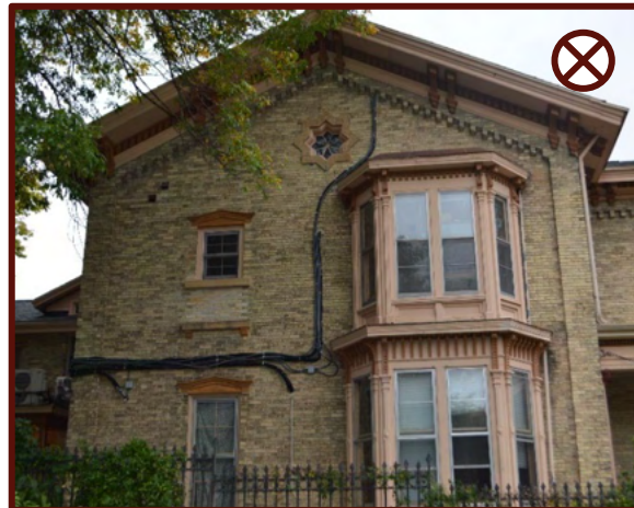
Figure 69: Example of inappropriately located utilities on a residence.
