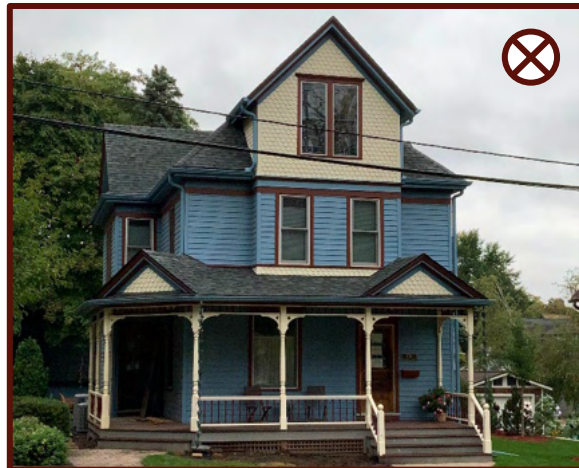
Figure 79: Inappropriate rooftop dormer addition with incompatible massing, height, scale, and proportions.
