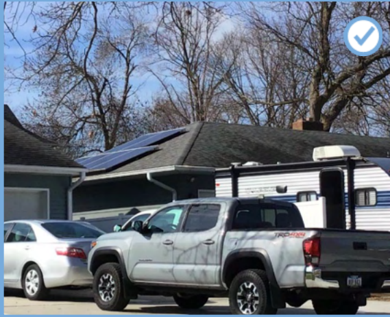
Figure 70: Example of appropriate location of solar panels on the side elevation of a roof.
