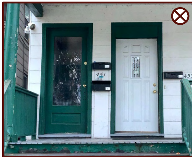
Figure 56: Comparison of a preserved original door (left) next to an inappropriate replacement door (right) on a historic residence.
