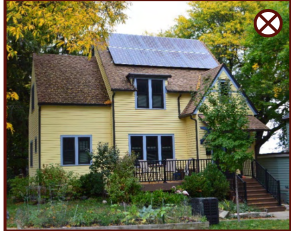
Figure 71: Example of inappropriate location of solar panels on the front of a roof.
