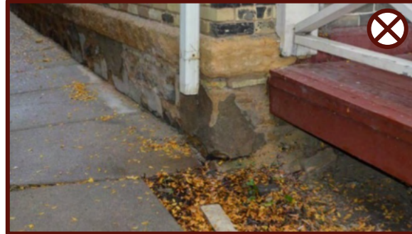
Figure 51: Example of inappropriate gutter, causing damage to the masonry.
