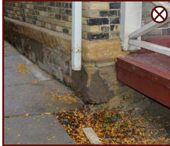
Figure 97: Example of inappropriate gutter, causing damage to the masonry.
